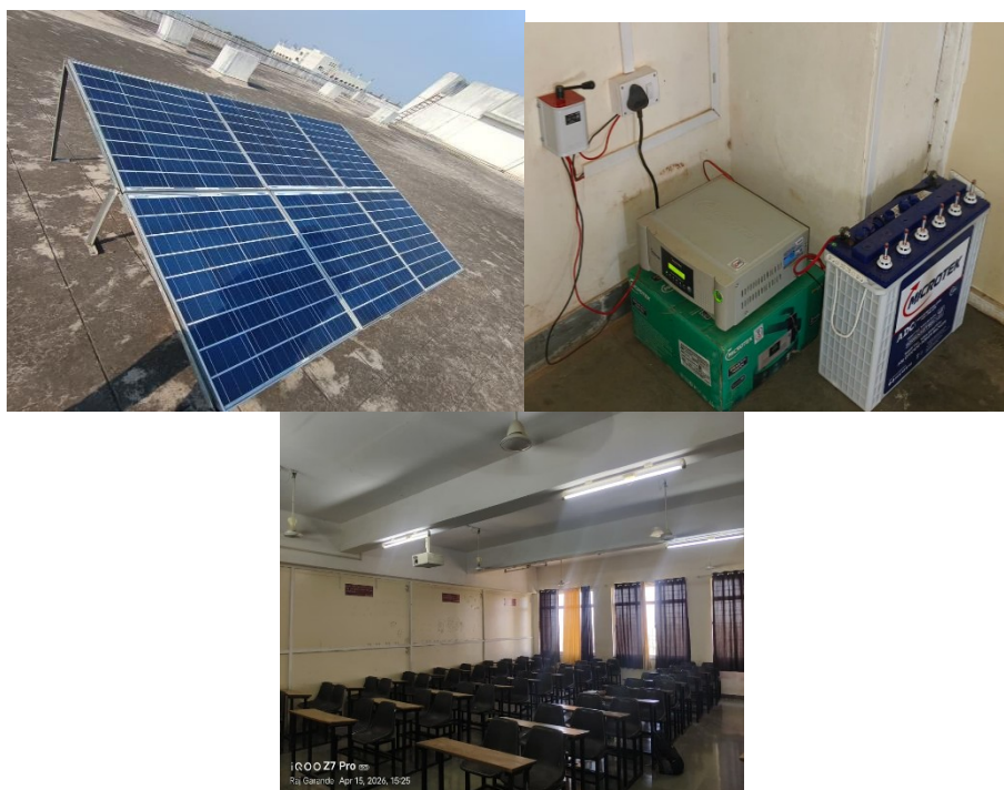
Fig. 2 Solar Panels, Inverter, Battery and Connected Loads
